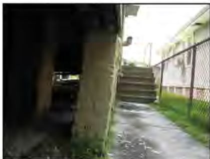
Structure No. 29: Tilted Piers
