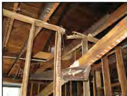
Structure No. 12: Termite Damage
