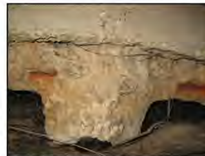
Structure No. 6: Scour Damage
