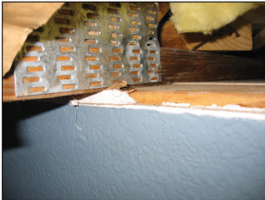
Truss bearing on a wall not designed as load-bearing.
