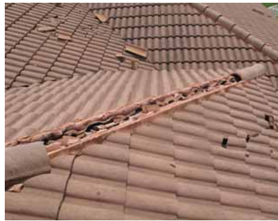
Figure 1: Displaced/fractured concrete hip tiles with adjacent fractured concrete field tiles
