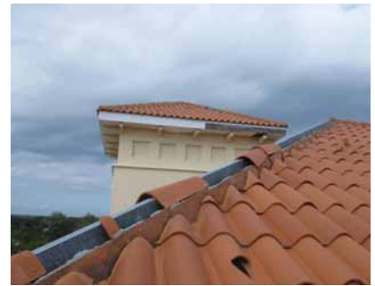
Figure 2: Displaced/fractured clay hip tiles with adjacent fractured clay field tiles
