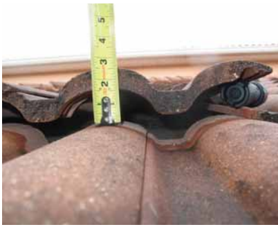
Figure 9 (above): Upward displacement at the leading edge of field tile under pressure
