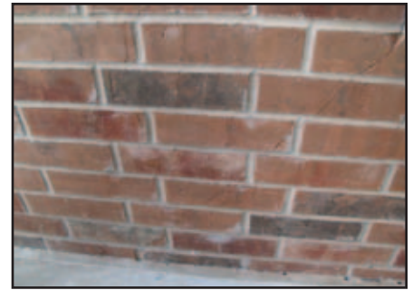
Figure 2: Diagonal fractures with no spalling
