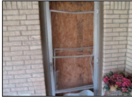
Figure 12: Fractured glazing and inward deformation of window frame
