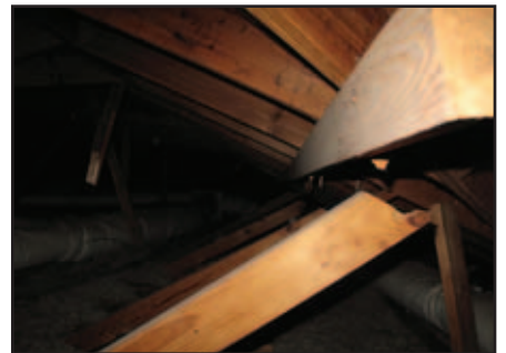
Figure 6: Fractured vertical strut along ridge and separated purlin supports
