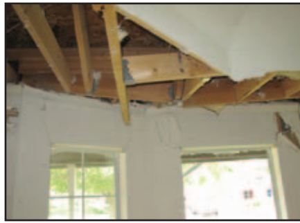
Figure 10: Collapsed ceiling finishes at area of displaced ceiling framing
