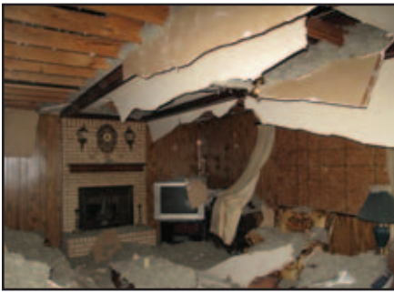
Figure 9: Collapsed ceiling finishes at vaulted ceiling with fractured rafters
