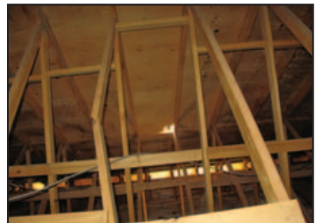
Figure 8: Compression fracture in truss web member
