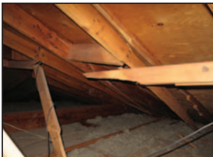
Figure 7: Fractured rafters and purlin
