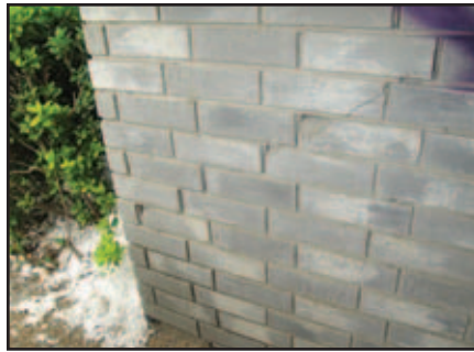
Figure 1: Diagonal brick fractures with spalling along brick edges
