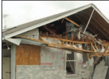
Figure 3: Displaced brick veneer with downward deformation of top plate
