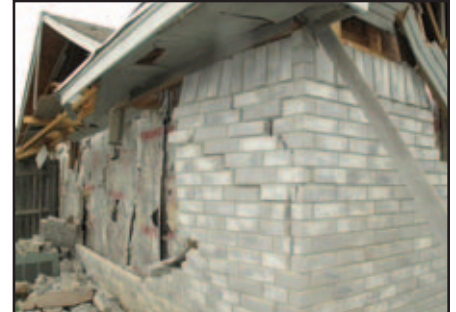
Figure 4: Buckled brick veneer with adjacent displacement of roof eave
