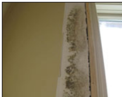
Figure 1 – Fungal growth behind removed wood trim.
