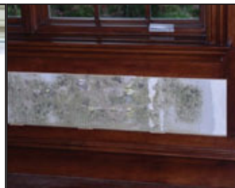
Figure 2 – Fungal growth behind wood paneling.
