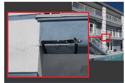
Figure 5: Stucco veneer distress at balcony beam and column interface
