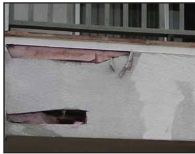
Figure 3: Removed stucco veneer
