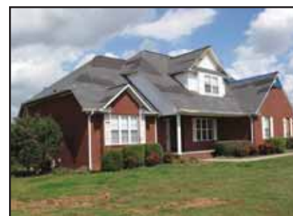
Figure 4 – Minimally damaged structure (DI #2, DOD #4)
