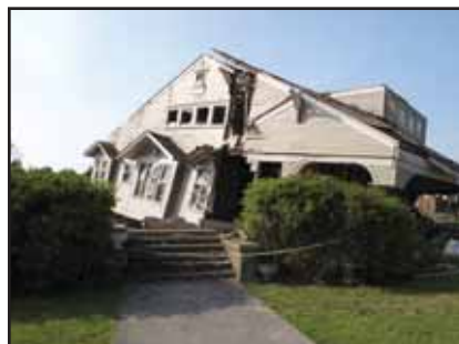
Figure 3 – Severely damaged structure (DI #2, DOD #9)
